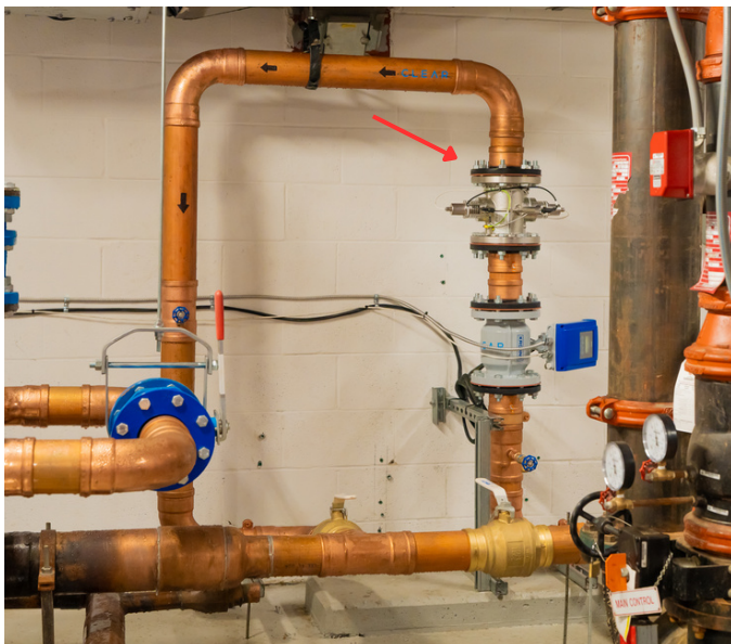
Figure 2. View of the RS104 UV reactor (red arrow) in the pump room.
