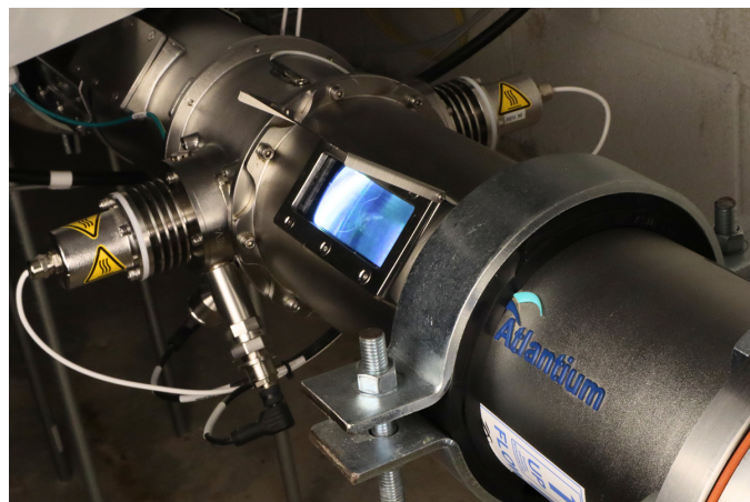
Clear's UV system, installed at Oscar Residences.
