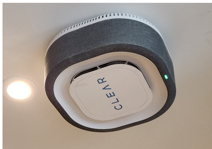
Clear's air purification, installed on the ceiling at Oscar Residences.
