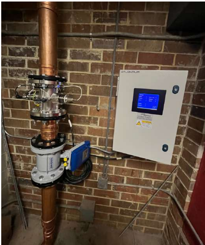
The pump room at Huntington Towers, showing the new UV water purification system (arrow)
